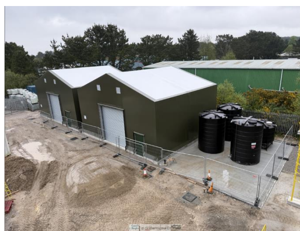
Figure 2: A photograph of the exterior of the 100-tpa lithium extraction plant during construction.
