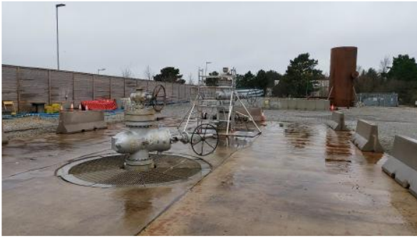
Figure 3: United Downs Deep Geothermal Power Plant wells UD-1 and UD-2
