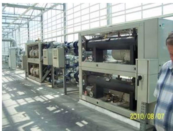
Figure 13: Heat pumps Daikin EWWD 440MBYN at the Greenhouse Complex “Berestyie”.
