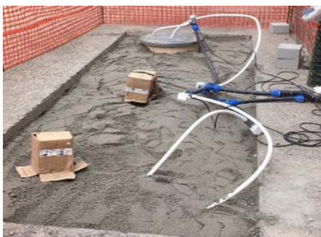
Figure 5: Refilling of the test site with a sandy layer at the top.
