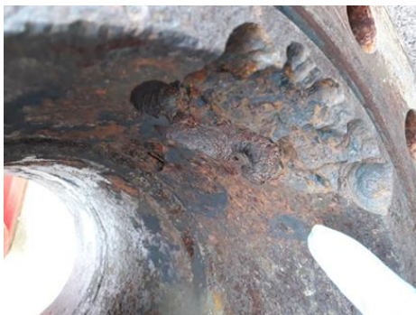
Figure 8: Localized corrosion on the reinjection pipe at Rittershoffen plant.
