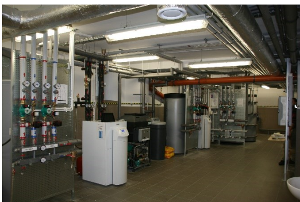
Figure 2: Research installation with heat pumps.
