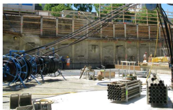
Picture 1: Jansen vertex 50 mm double-u loop installation into borehole field in Uster, CH.
