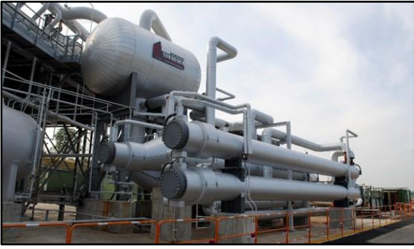
Figure 4: Soutz-sous-Forêts geothermal plant
