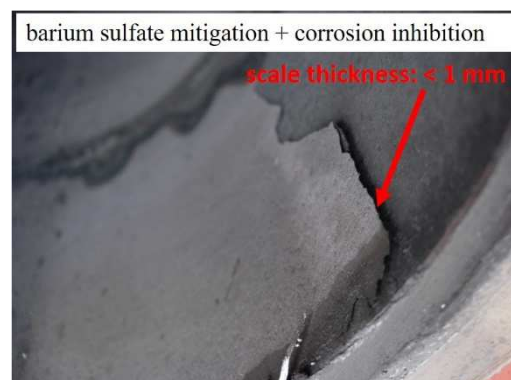
Figure 10: Scale deposit inside the monitoring pipe with injection of the barium sulfate antiscalant (Reference Inhibitor) in combination with the corrosion inhibitor (Additive 3) after 4 months exposure.
