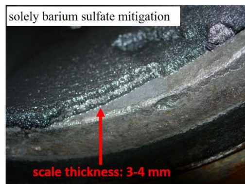
Figure 9 Scale deposit inside the monitoring pipe with injection of the barium sulfate antiscalant (Reference Inhibitor) after 4 months exposure.
