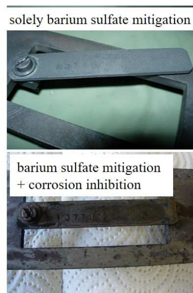
Figure 13: Top: Coupons after exposure to brine treated only with barium sulfate antiscalant. Bottom: Coupons after exposure to brine treated with barium sulfate antiscalant and corrosion inhibitor.
