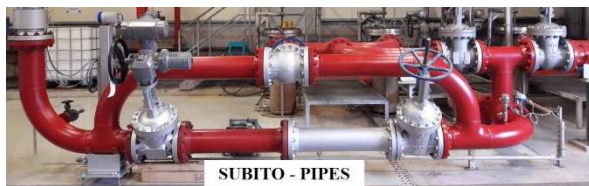
Figure 7: Pipes of the return line for scale monitoring at the geothermal site of Insheim.
