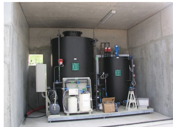
Figure 6: Station for water decalcification and inhibitor dilution (EDA RENOVÁVEIS).
