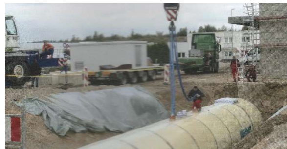
Figure 3: Placing of a 100 m 3 low-temperature storage tank at oeding print GmbH (photo Ostfalia).
