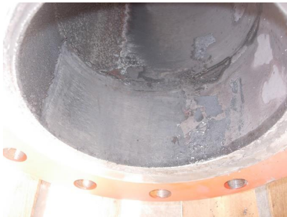
Figure 8: Scale deposition within the monitoring pipe the other geothermal site.
