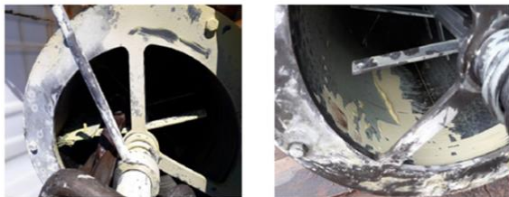
Figure 11: Production filter clogging: interaction between brine and scaling inhibitor at high temperature at Soultz-sous-Forêts plant.
