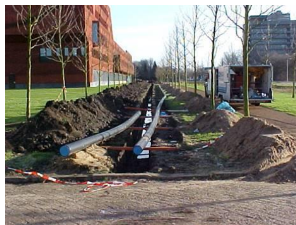
Figure 3: Construction of low temperature grid at the University of Utrecht. Source: IF Technology.
