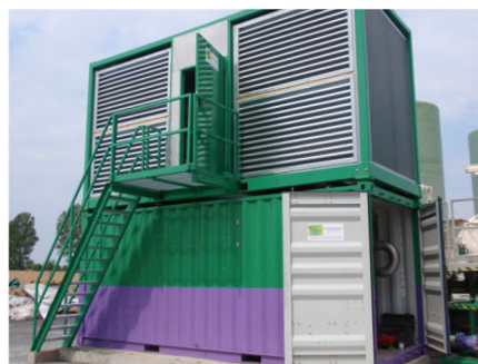
Figure 5 : Mud cooling system
