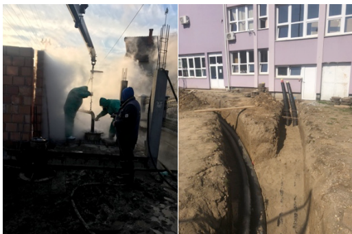
Figure 3: Construction of the GeoDH system in Bogatic; operation on the well head; pipe line
